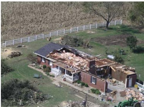
Tornado Damage in Southeast Missouri after severe storms of September 2006.
