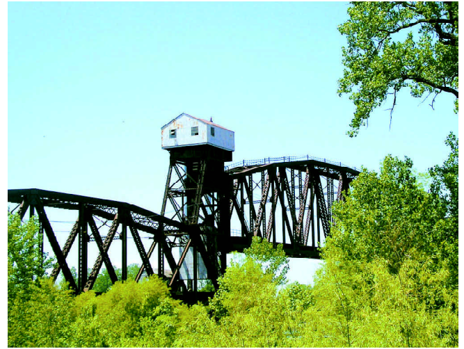
Above: The historic Boonville bridge showing the bridge house. Photo courtesy of Theresa Krebs.
