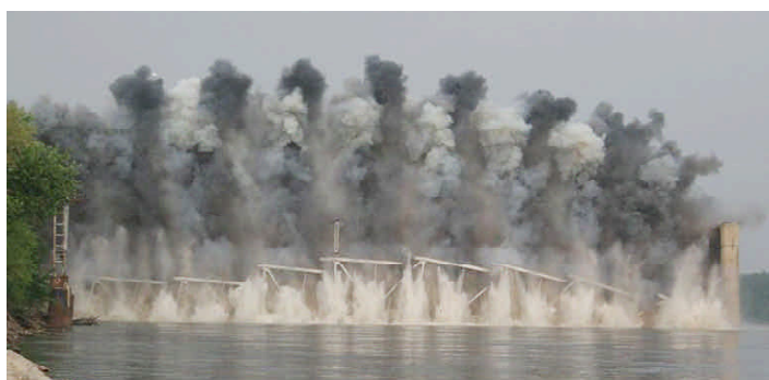
Left: This stunning sequence of photos, taken by Pat Larkin of L & L Photography, shows the Waverly bridge in its last moments as a demolition crew brought it down to make way for a new span.
